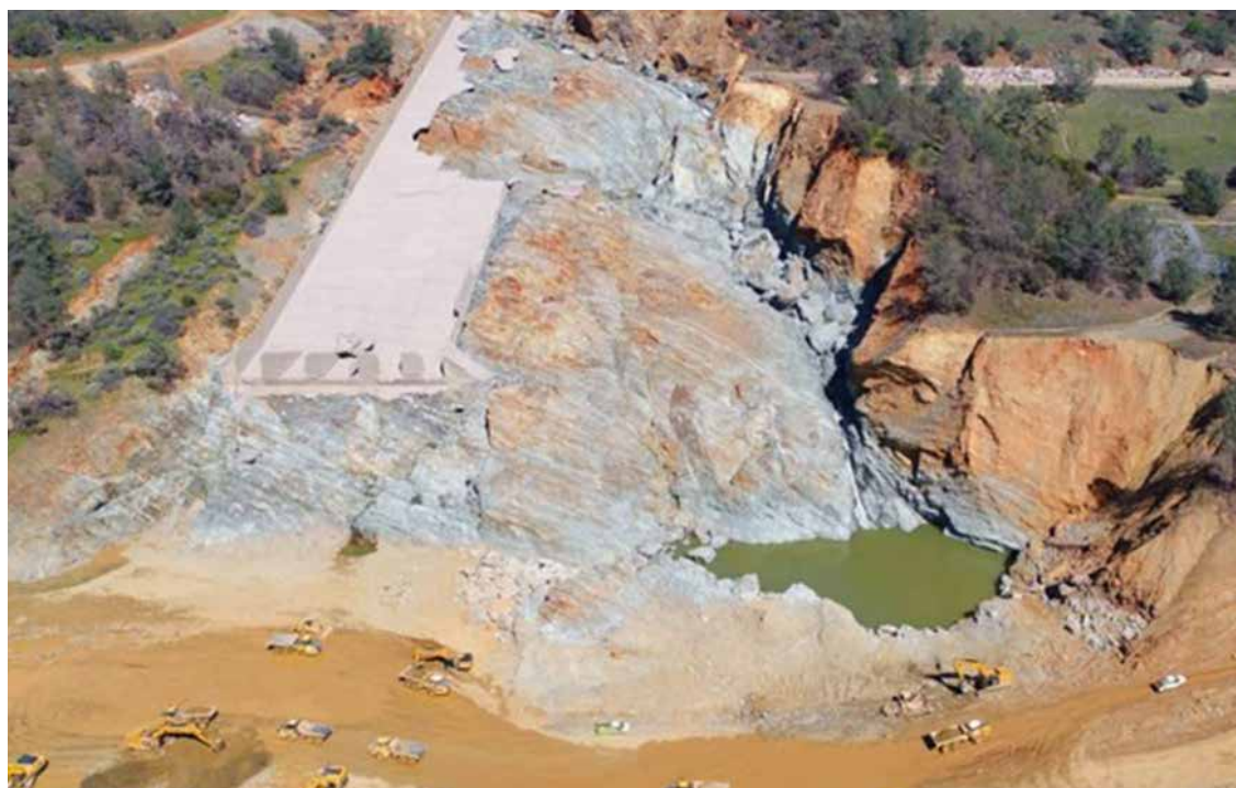
Oroville-dammens utskov efter haveriet 2017. Foto: California Department of Water Resources.
